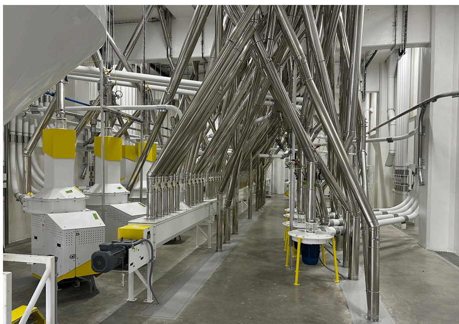
WEAVE OF PIPES: After starch and Pentosane streams are separated, the protein extracted is dried in ring dryers, converted into granular form and sent to the packaging operation.
